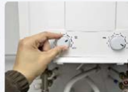
Optimising Boiler Flow Temperatures
